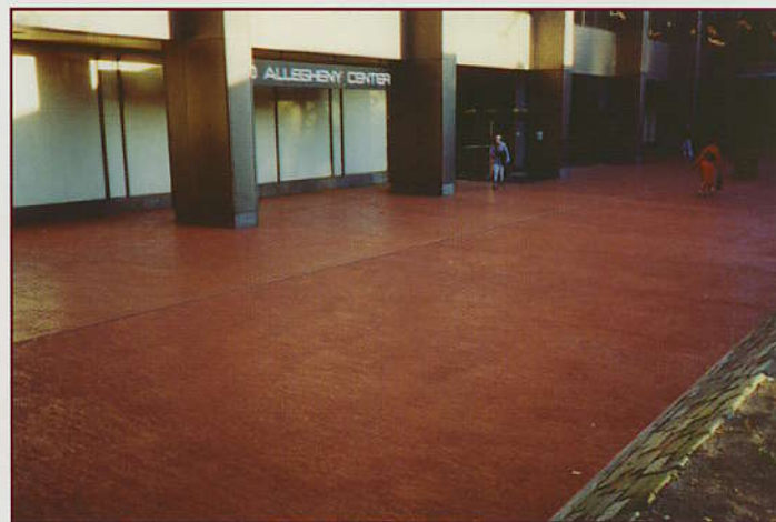
A tough PERMA•CRETE ® coating over this worn concrete plaza at Pittsburgh's Allegheny Center added a smooth finish and color to the project.
